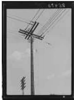
Figure A.131: Telephone lines in rural Virginia (from LC)
